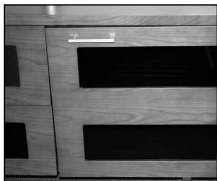
INCORRECT! Door is out of alignment with the rest of the unit.
